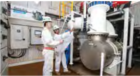
Sembcorp Marine engineers inspecting the Semb-Eco LUV Ballast Water Management System
