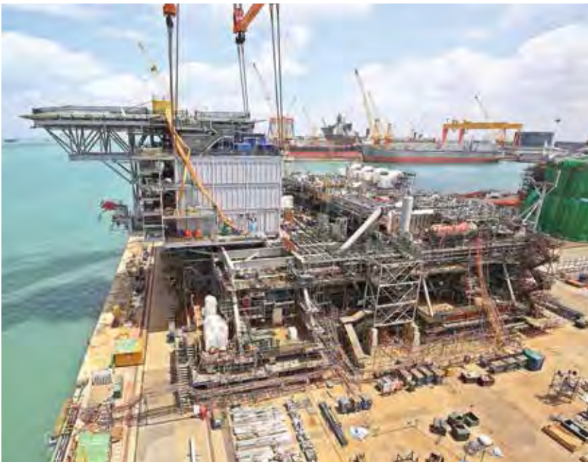
Shell Vito FPSU topside and living quarters under construction at Sembcorp Marine Tuas Boulevard Yard
