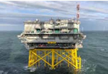
Hornsea Two Offshore Substation Platform for the world's largest offshore wind farm, Hornsea Two Offshore Wind Farm
